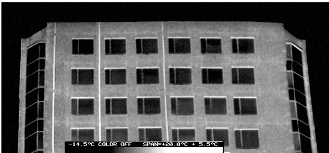
Figure 10. Negative Building Pressure (-60 Pa), T_o = -7^{\circ}\text{C} , maintained for a duration of 4 hours prior to inspection.
